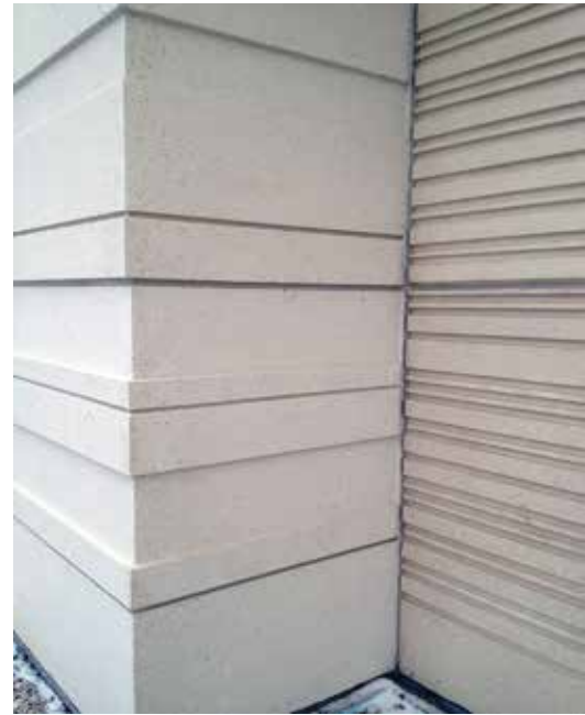
Entries feature 1-inch-thick reveals, producing a ribbed pattern that provides color and dimensional contrast to the other finishes. Photo: Gage Brothers Concrete Products.
